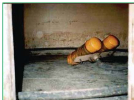
After HydroLock Degassing and Cleaning
